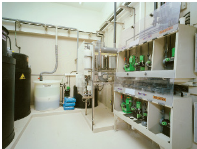
Installation de dosage, STEP Neuchâtel
